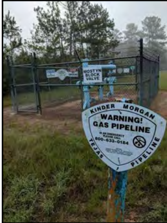
19 : PIPELINE STATION ON SITE
