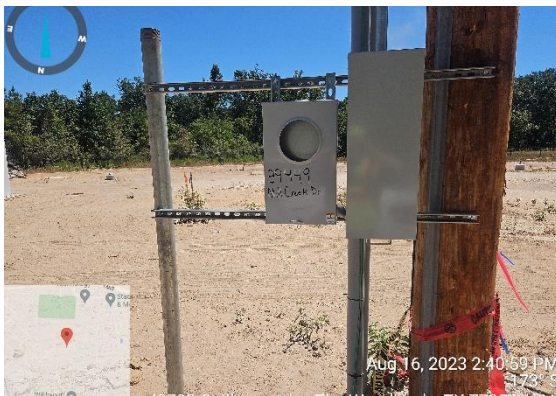
Electrical service entrance
