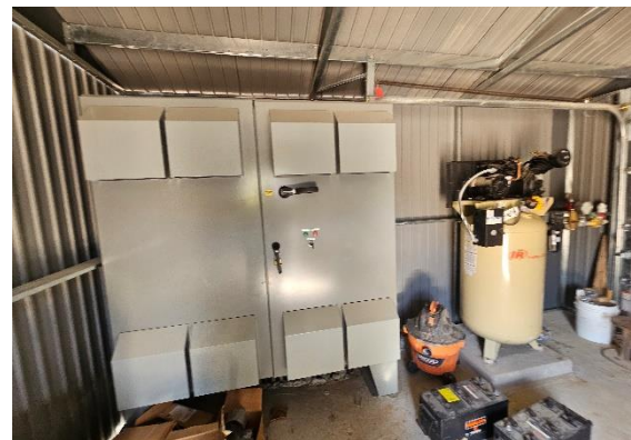
VFD and air compressor
