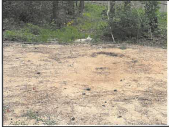
Address settlement at SH 249 crossing exit pit.
