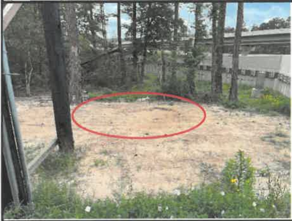
Address settlement at SH 249 crossing exit pit.
