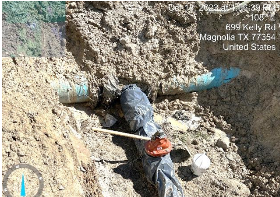
Well Discharge Piping Tee to Future GST
