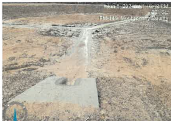
Detention pond with silted pilot channels
