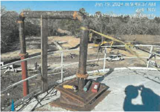
Fill line piping
