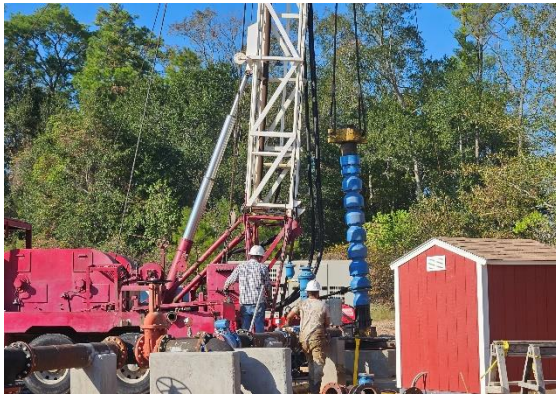
Permanent pump installation
