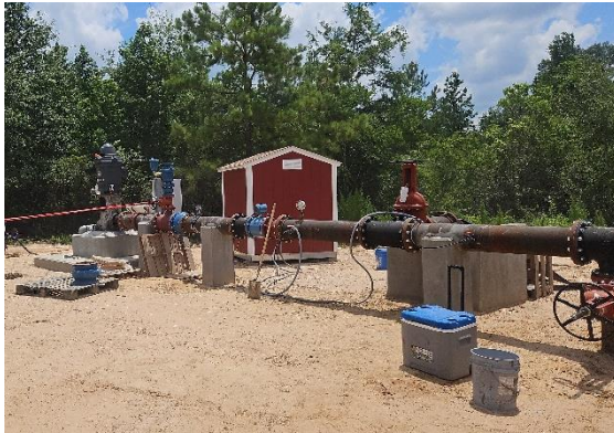
Water well discharge piping
