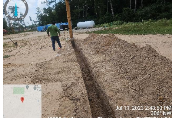
Electrical duct bank to power pole
