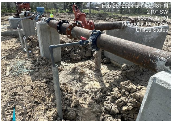
Water well discharge piping and chemical injection
