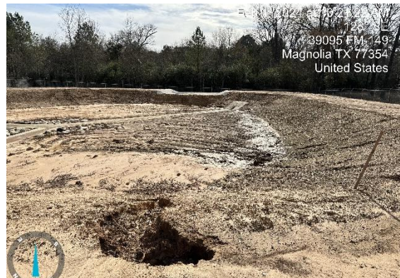
Detention pond erosion
