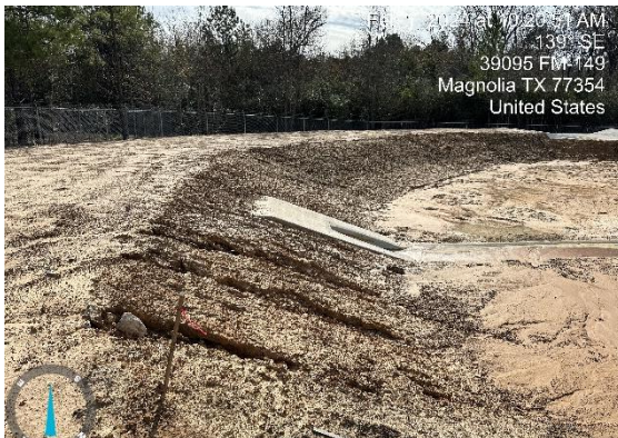
Detention pond erosion
