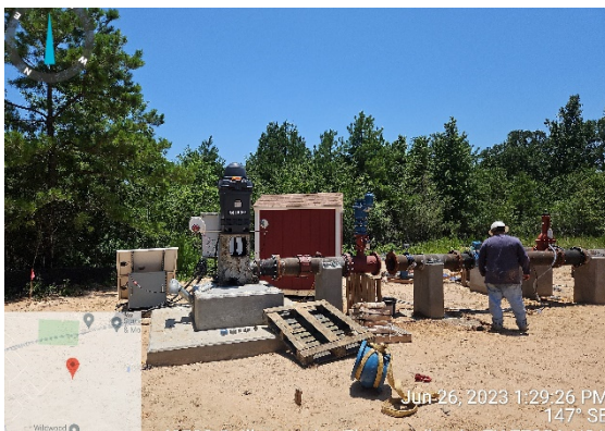
Water well and discharge piping
